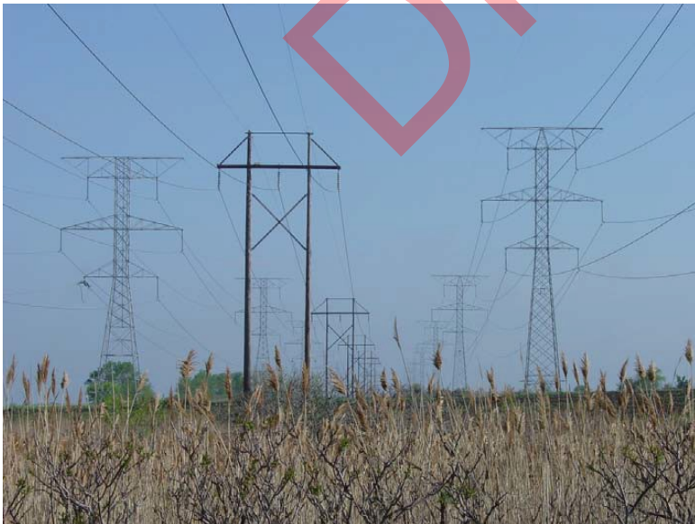
Multiple Lines in a Power Corridor. The lattice towers are twice the height of the wood pole structures. (Source: Argonne Laboratories staff photo)
