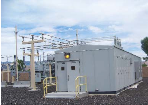
Fairview Substation, Carson City
