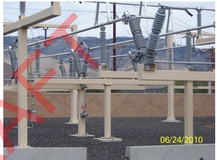
Fairview Substation, Carson City
